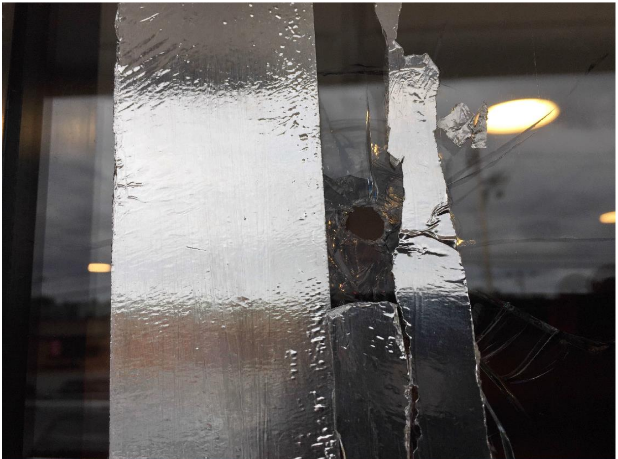
Exterior view of glass window with bullet hole (employees placed tape around damage to minimize the potential of glass falling away).
